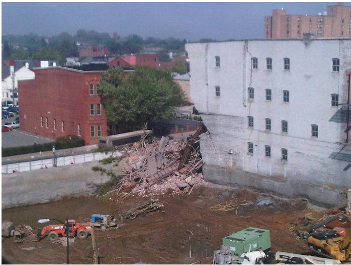
The Lancaster Museum of Art building after a portion of the building collapsed onto an RRTA bus heading to Queen Street Station on Queen Street.
