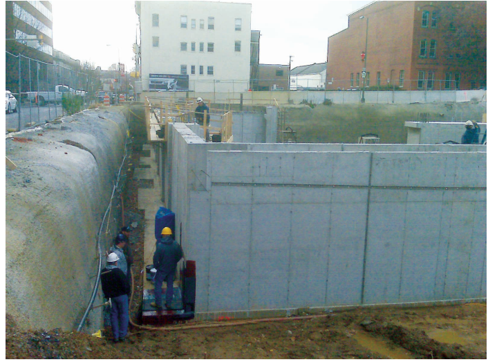
Foundation being constructed for Queen Street Station Phase II on the corner of Queen and Chestnut Streets in Lancaster City.
