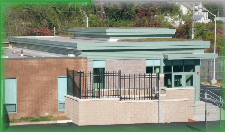
A green roof to help with energy savings and reduce storm water runoff.
